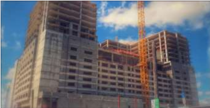
Margaratville is going UP. We have heard that construction on the beach side of the building will start in January and may require a few months closure of the music shell. Go get your music fix now!
